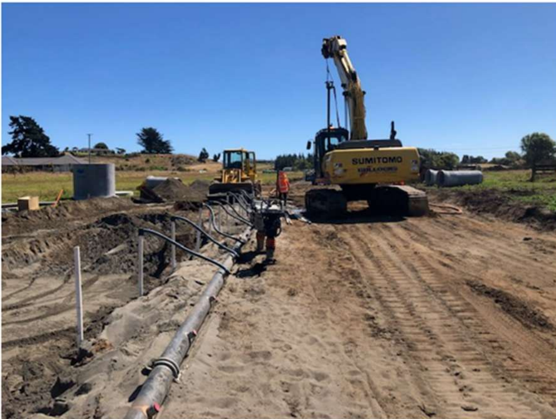
Photo: Fitzherbert Avenue Construction - Heavy storm water pipes and manholes being constructed underground. Dewatering taking place.
